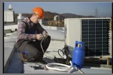
Corporate Ductable AC Installation Service
