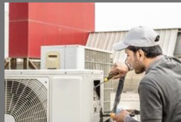
HVAC System Maintenance Service
